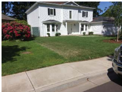
The storm drain relocation was completed well within the 30-day construction schedule.
