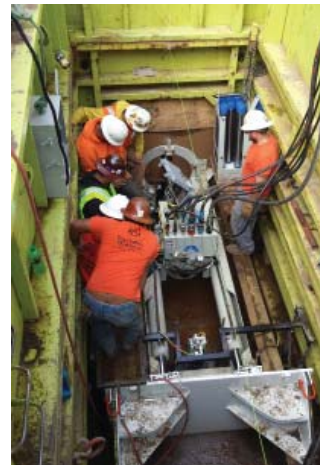
The boring equipment fit snugly in the bore pit. The team successfully bored the smaller pilot bore and then placed the larger 20-inch steel casing - all within one weeks time.
