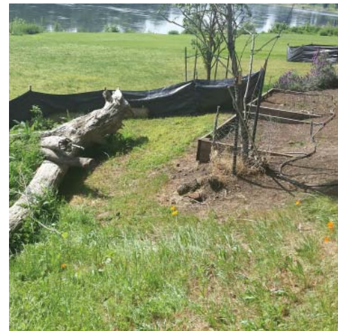
The new outfall location had to be designed into the existing landscaping. The team worked around planter boxes and worked carefully to avoid impacts to the floodplain.
